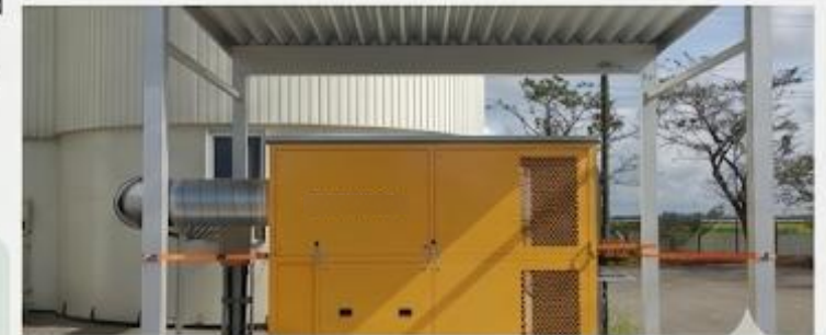
INSTALLED UNIT: Site conditioning for a silo. Note: The 'GRANIFRIGOR' brand and external ducting.
